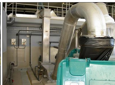
Press washer with compacting screw and washing of screenings
