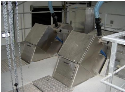
Fine screen in channel stairs screen
