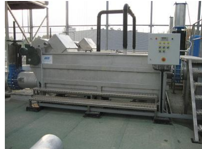
Fine screen in stainless steel tank
